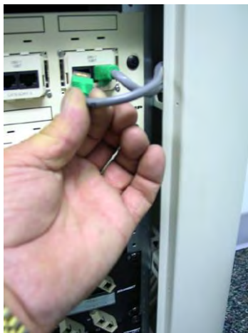
LDS with Patch Panels and Data Cables connections by others.
