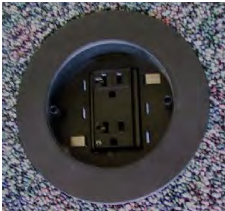
Completely Installed Electrical Outlet ( Top View )
